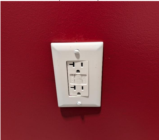
Photo #13 – Cover plate not fully screwed on.
