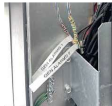
LABELS AT GENERATOR
